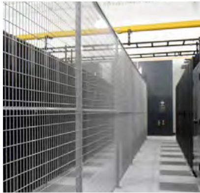
Private Cages An added layer of physical security to protect your digital assets
